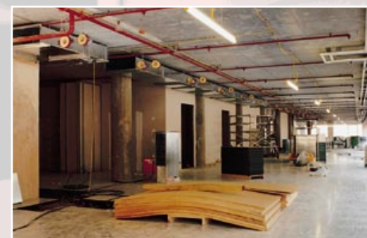
By April, the ceiling space is looking very busy indeed. The air-conditioning ductwork is lagged, air and water direction noted and
