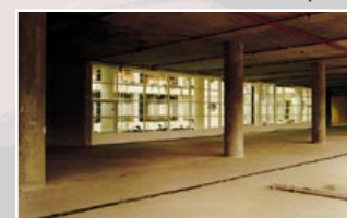
Note the extensive sprinkler system pipework in the ceiling area.
