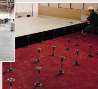
Note: the level of the false floor is much higher here than in the general office area, enabling safe housing of the cabling required for provision of voice and data services.
