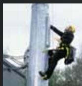
Vodafone, Southern England
